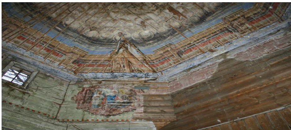
Fig. 5. Wall polychrome of the church in Miękisz Stary, visible illusionistic representation of the open sky placed in the dome above the architectural entablature and the figures of the Evangelists in the pendentive; photo T. Tomaszek.
