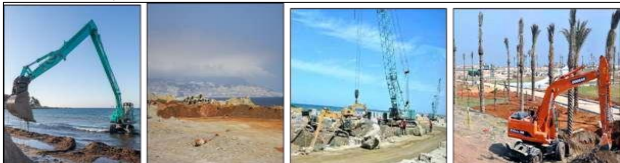
Figure 06: Photos of Ecological Depollution of the Site During Construction (Source: Project Construction Company MEDITRAM).
