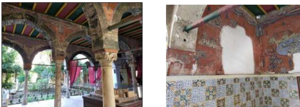
Figure 6. The Noted Deterioration in Ahmed Bey Palace (Note: By Nadira Bouguebs, 2025)
